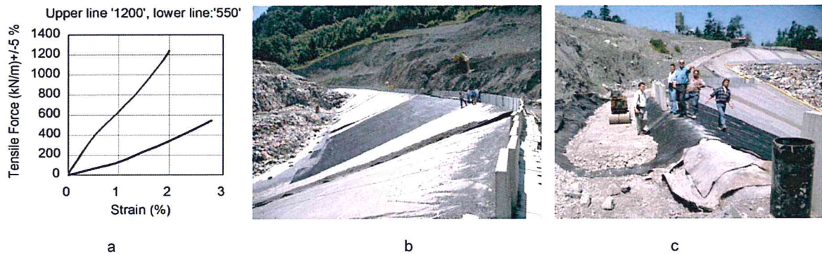
Figure 3. a: tension vs. strain for the aramid geogrids used in 1995-1996; b: installation of geogrids on the first partial slope; c: heavy anchoring trench due to the high tensile forces
